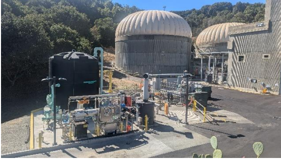
10/3/2024: Upgraded Receiving Station
