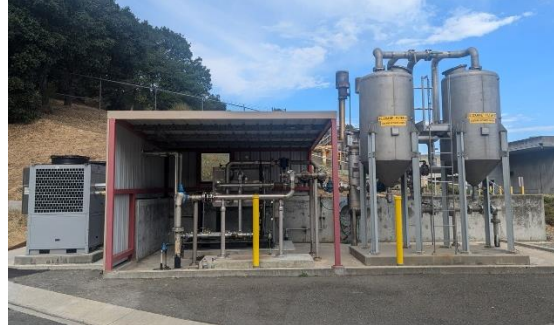
2/13/2025: Upgraded Biogas System
